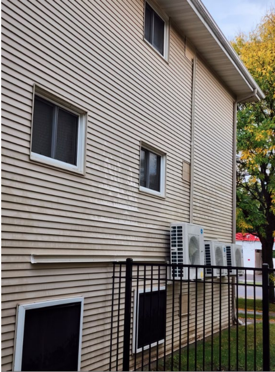
Figure 9. Outdoor unit placement at MF_61
