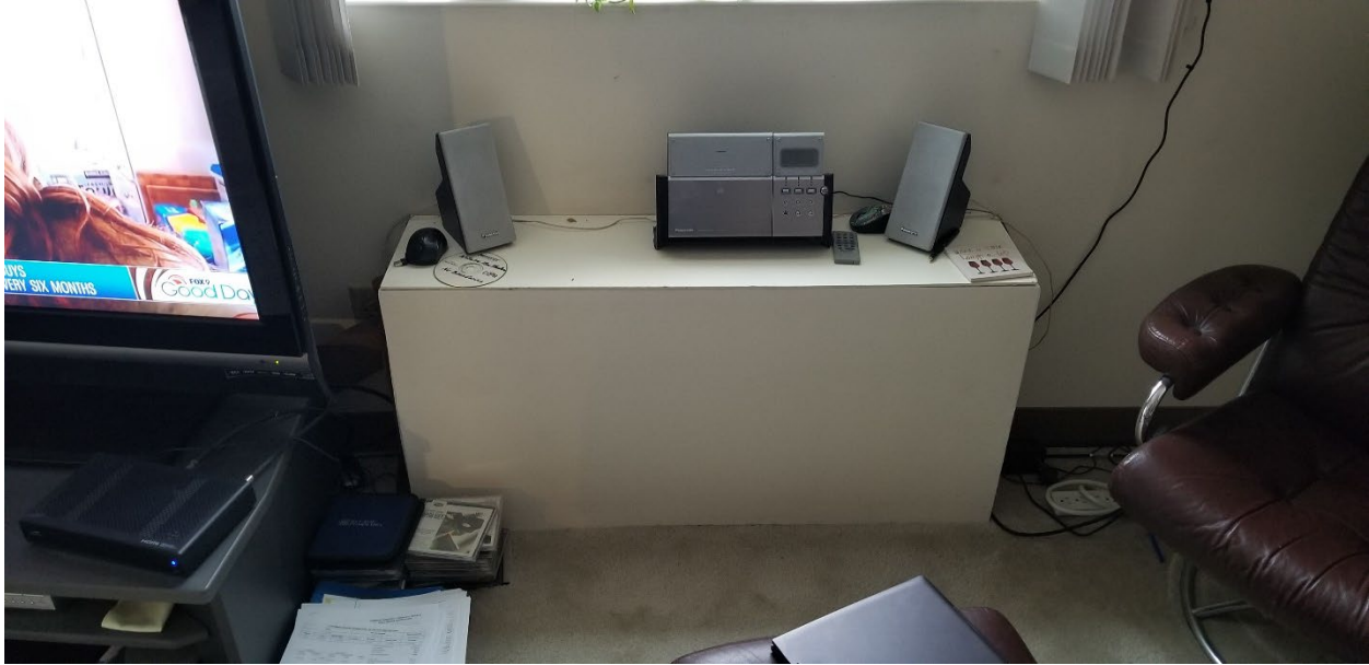
Figure 7. The existing PTAC heating system in the living space of MF_60
