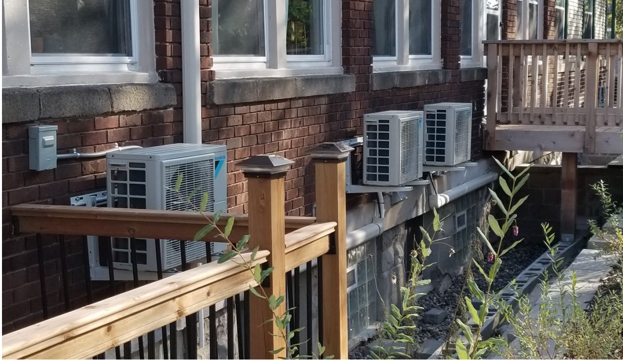
Figure 10. ASHP outdoor units at MF_7
