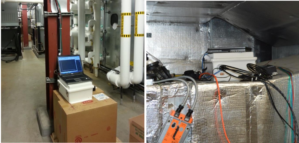
Figure 13: Logging equipment left on site for recording and transmitting measurements
