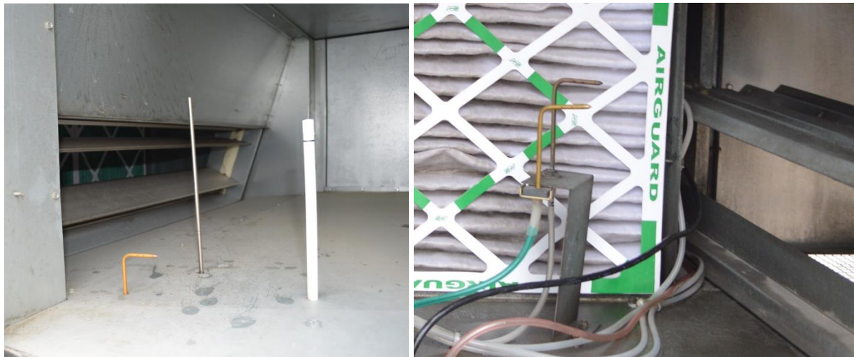
Figure 11: Supply T/RH sensor and static pressure sensor co-located with automation system sensors
