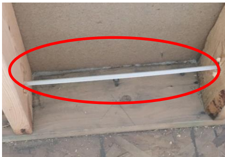
Bottom plate/sheathing gap
